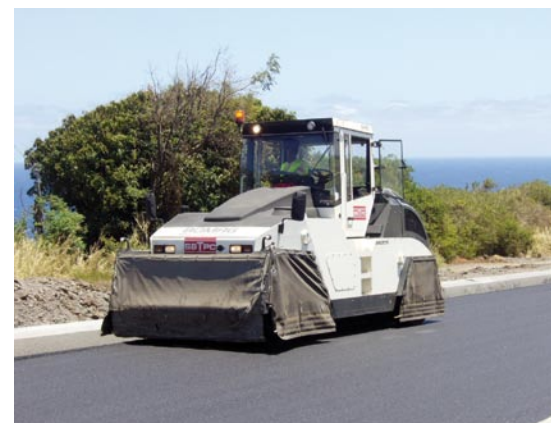
Pneumatic tyred roller with "skirts" to keep tyres warm during compaction to prevent asphalt from sticking.
