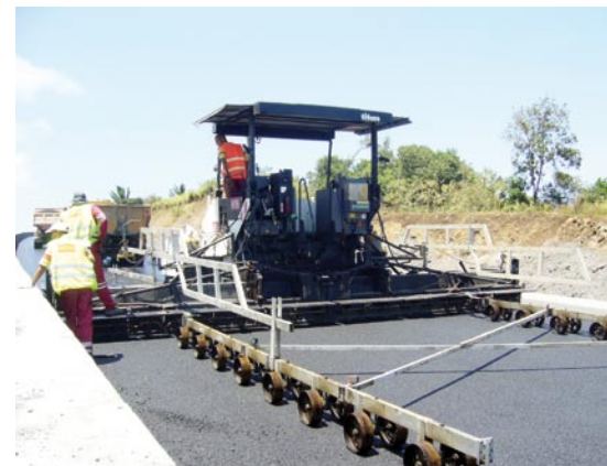
A Titan paver paving HiMA with a rolling straight edge to improve riding quality of the asphalt.
