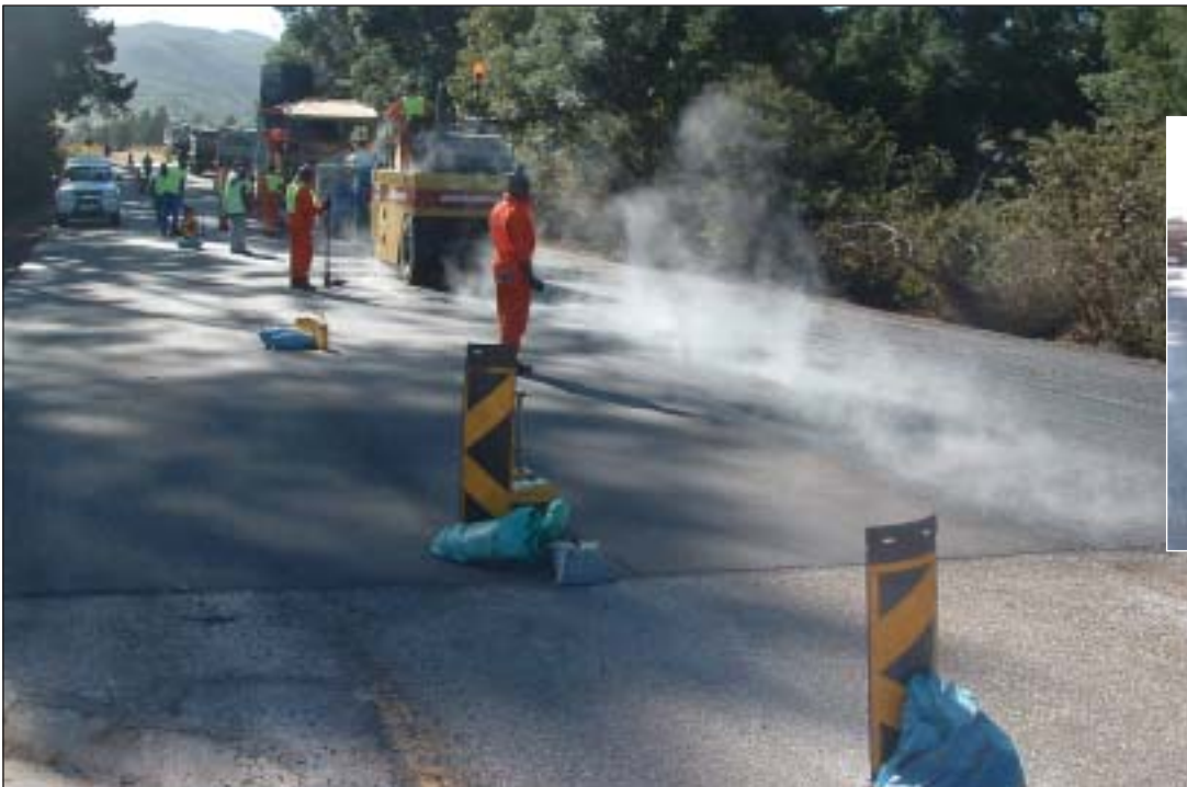
Steam rises from a newly paved section of the Gamtoos/Van Stadens project.
