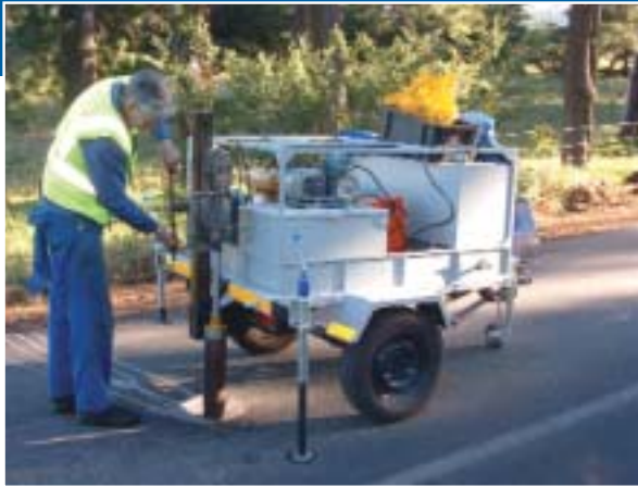
Much Asphalt's Jimmy Henderson cuts cores to check the density of the resurfaced pavement.
